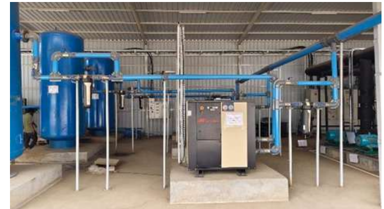
Compressor with Compressed Air Piping
