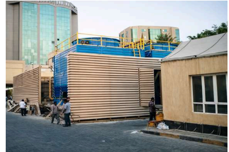
4 Cell Cooling Towers
